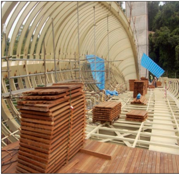
Figure 14. IJP and RSP Architects Planners and Engineers, Henderson Waves, Singapore, 2008 Timber deck of the main span under construction. This central arch spans 57 metres (187 feet), and rises to more than 6 metres (19.6 feet) at its apex. Too large to be prefabricated off-site and craned into position, it was assembled on a makeshift platform directly above Henderson Road, then raised into position by a battery of hydraulic jacks. The centre-lines of the steel members shown (central arch, edge member, mid-height member and curved ribs) are determined by a single set of parametric equations.
