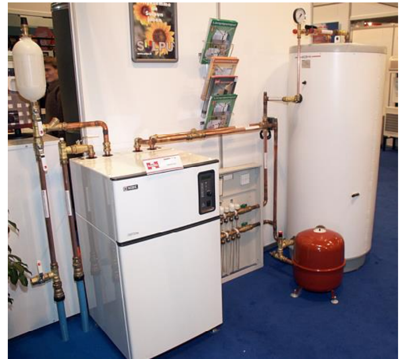
A ground-source heat pump plant
