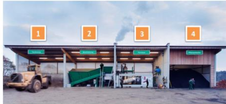
Greenlife Ressourcen GmbH, Hoberndorferstraße 21b, A-8230 Hartberg T. +43 3332 63374, office@greenlife.co.at , www.greenlife.co.at
