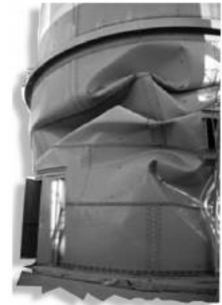
Axial buckling failure in service.
