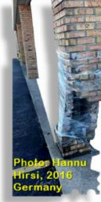
Loss of stability of a column. Original temporary reinforcement method.
