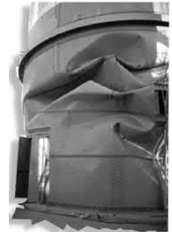
Axial buckling failure in service.
