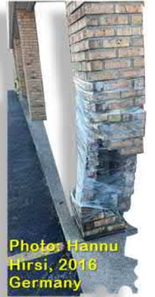
Loss of stability of a column. Original temporary reinforcement method.
