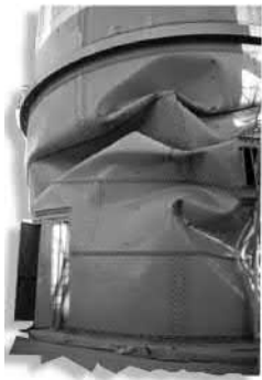
Axial buckling failure in service.
