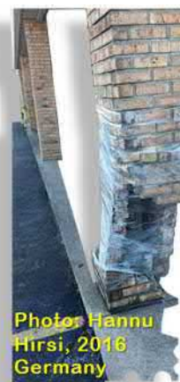
Loss of stability of a column. Original temporary reinforcement method.
