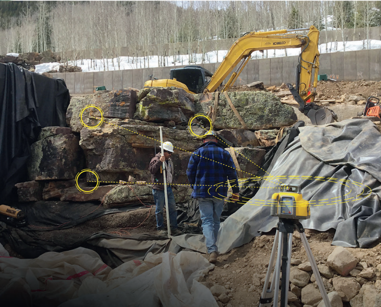
FIGURE 0.1.11 3D Boulders scanned and assembled in the computer for contractor construction Image: Design Workshop
