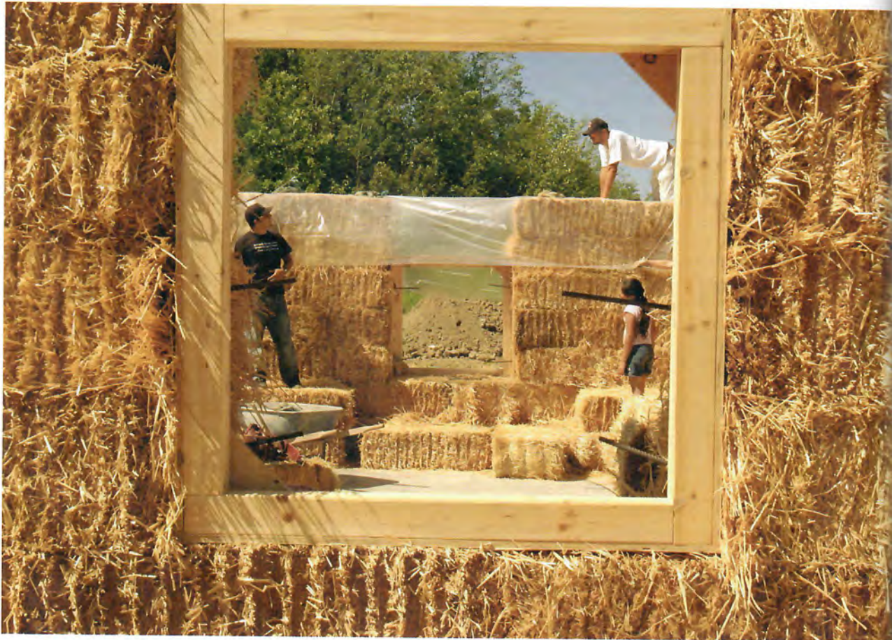
△ Straw bale house under construction, an example of Corum's work with Native Americans (photo: Skip Baumhower).
