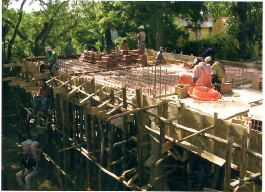
Figure 1.2 Construction workers prepare formwork and rebar for the reinforced concrete slab in Antananarivo, Madagascar
