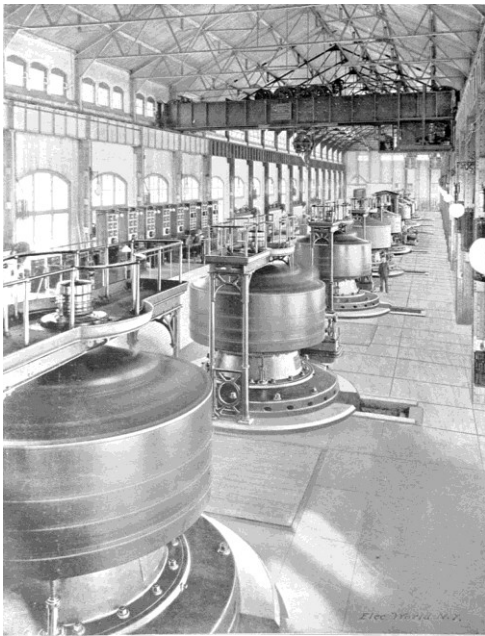
FIG. 11.—A VIEW OF THE TESLA ROOM, LOOKING SOUTH FROM THE VISITORS' GALLERY.
