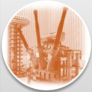
Voltage source (Transformer)
