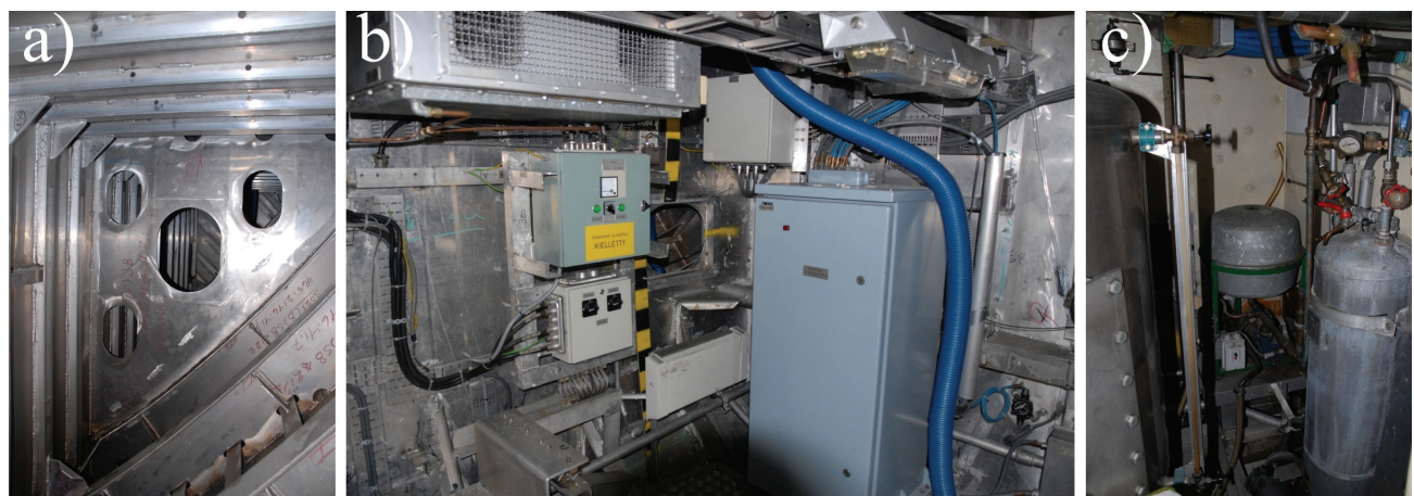
Figure 4: Flooded compartments: a) side tank with anti-sloshing bulkhead, b) equipment room and c) pump room
