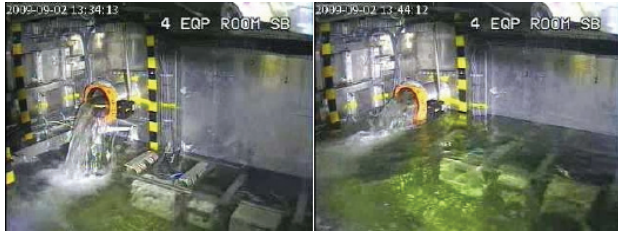
Figure 8: Different flow conditions of the valve between the side tank and the equipment room
