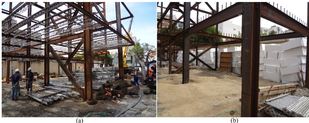
Fig. 2. Problems found in exploratory study 1: (a) inadequate location of steel component inventories and (b) a large inventory of thermal insulation parts.
