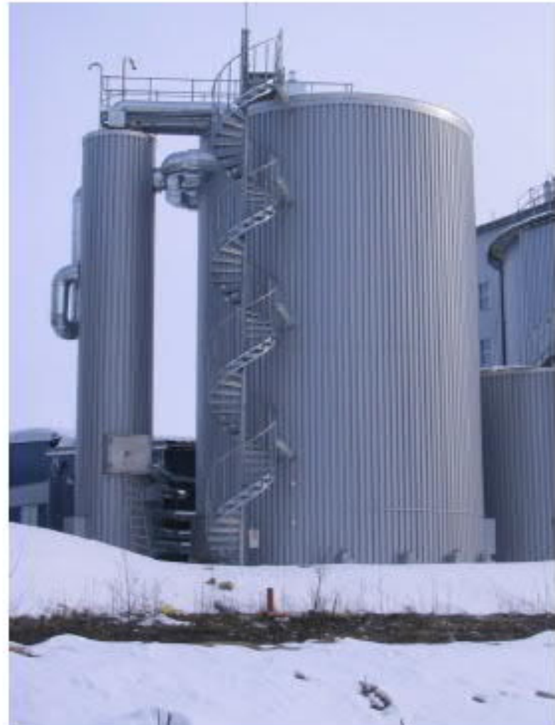
Typical Biobed® EGSB plant at Lapin Kulta, Haparanda (Finland)
