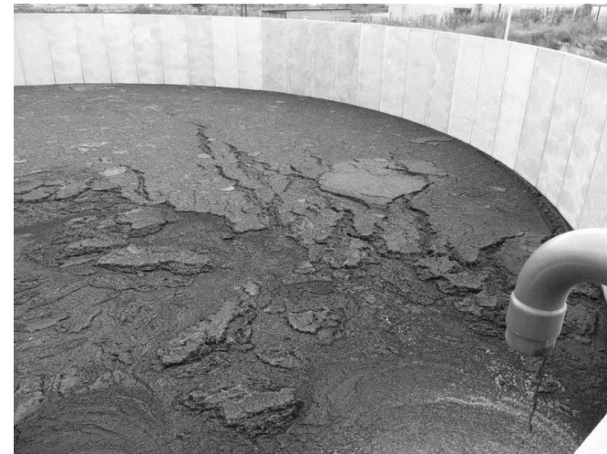
Digestate storage tank DOI: 10.5593/SGEM2015/B41/S17.046
