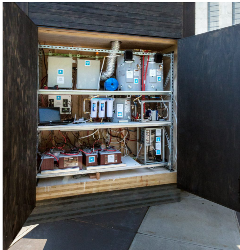
compact building service
