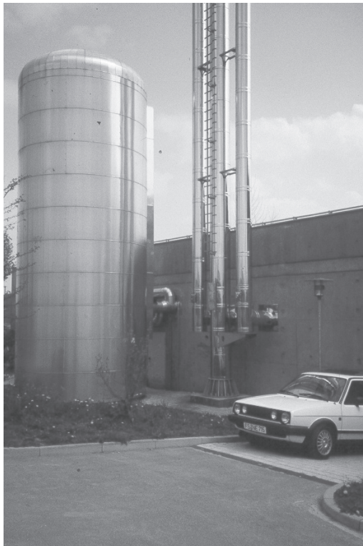
Figure 6.13 Buffer storage (100 m 3 volume) in the solar district heating in Neckarsulm.
