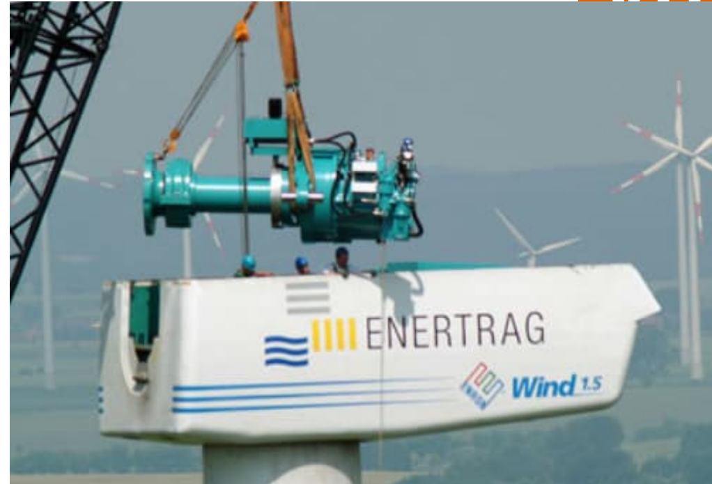
Gearbox and main shaft replacement in an old wind turbine Source: Windpower monthly
