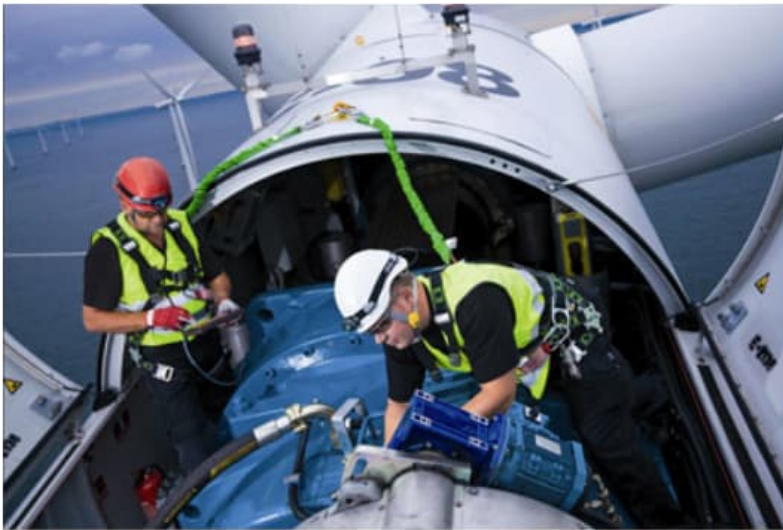
Servicing a gearbox in a modern geared offshore turbine Source: Windpower monthly
