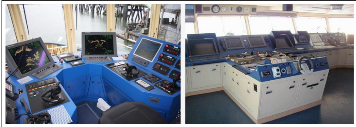
Figure 3. Ship bridge console of a tugboat (left image) and a large merchant vessel (right image).
