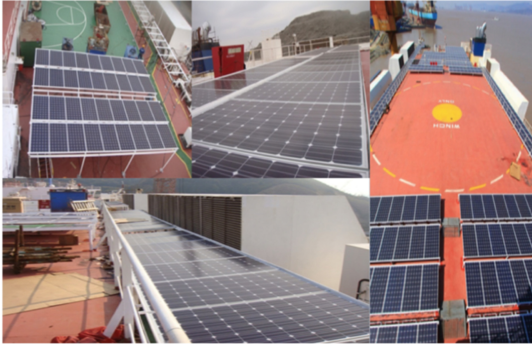
Fig. 5. A photo of the solar PV system installation on the actual ship.
