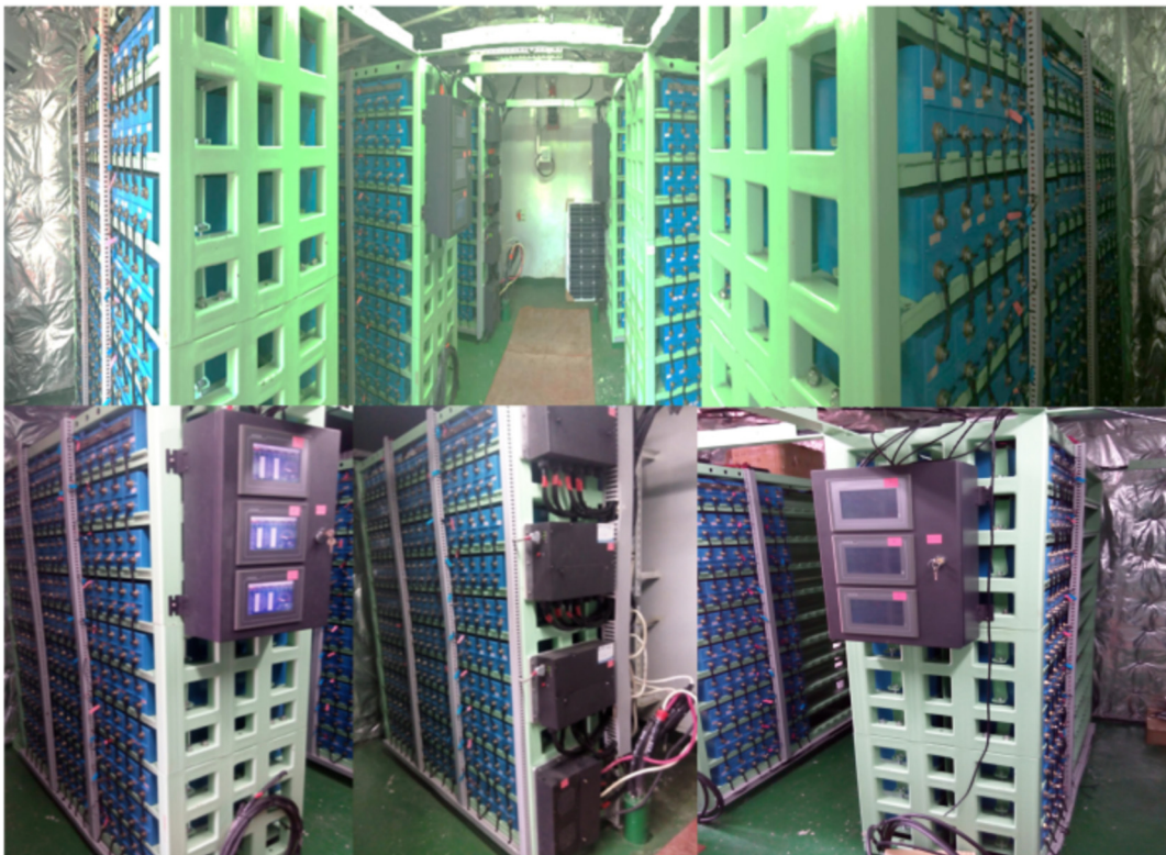
Fig. 6. The battery system installation on the actual ship.
