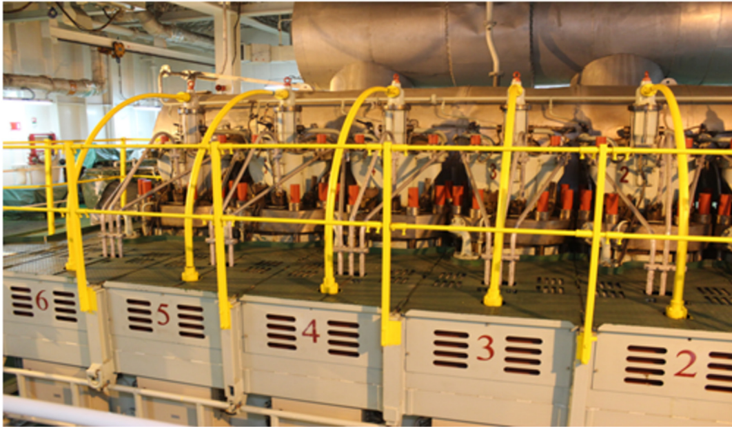
Fig. 7. A 3# diesel generator.
