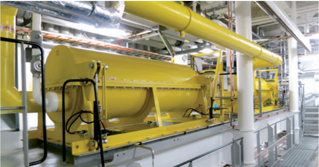
Wärtsilä Gas Valve Unit Enclosed Design (GVU-ED™) installed directly in the Engine Room
