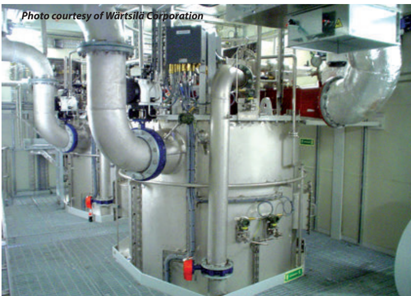
Inert Gas System
