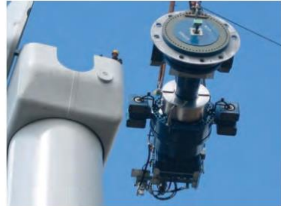
Figure 6.58 Lifting of gearbox and brakes of HAWT. (Courtesy of Paul Anderson through Wikipedia.)
