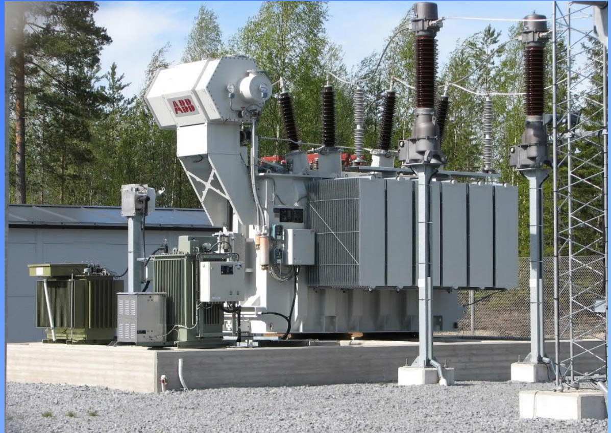
110 kV / 20 kV primary transformer
