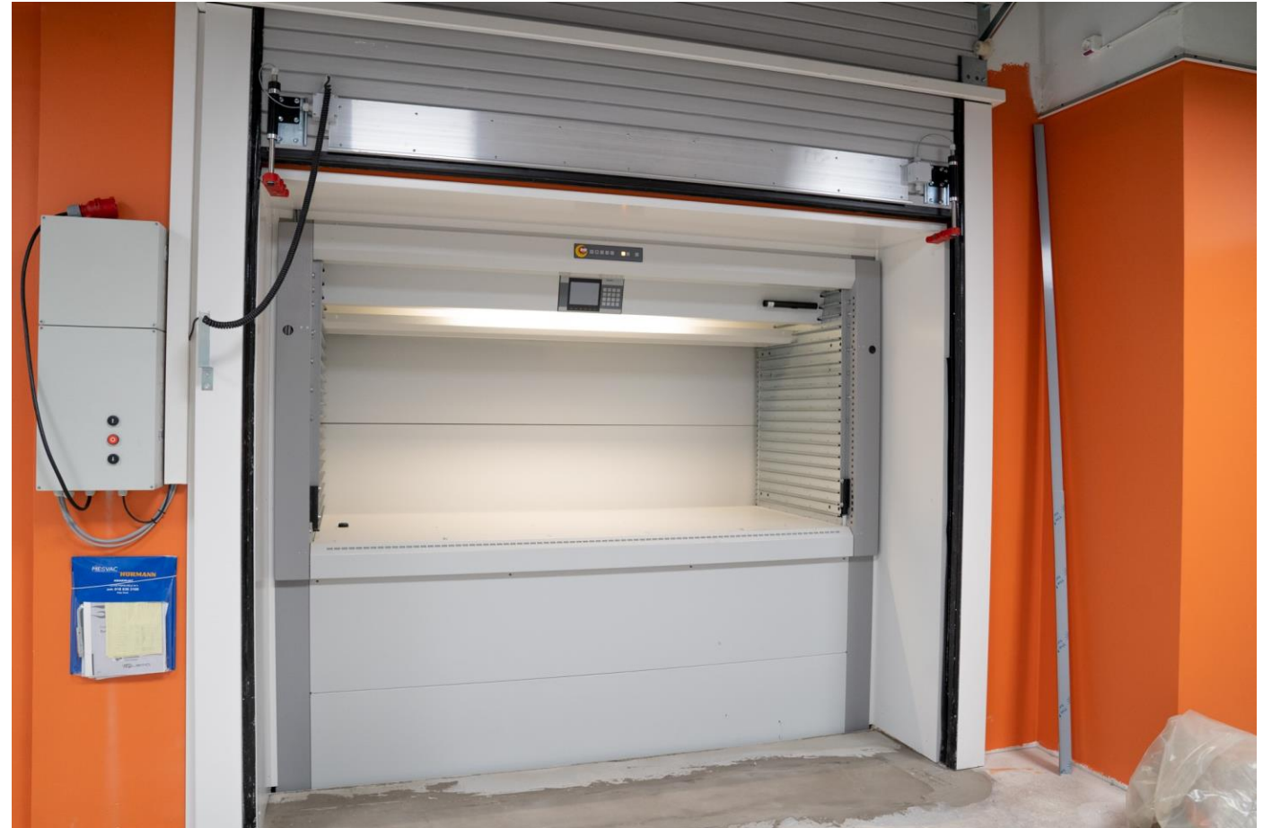
Kardex vertical storage in Kajaani hospital
