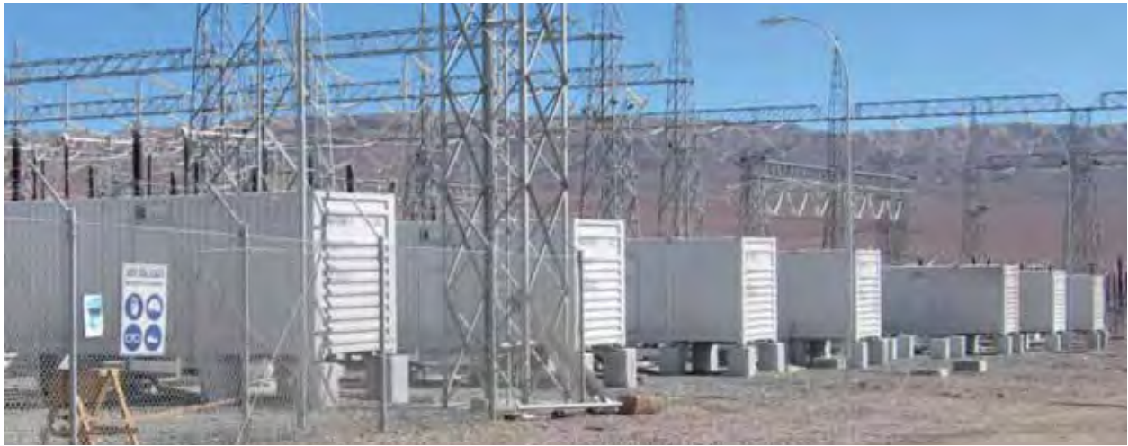
Figure 3-3 | Li-ion battery supplying up to 12 MW of power at Los Andes substation in Chile (A123, 2009)
