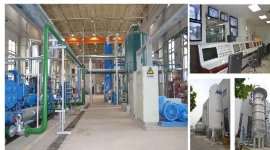
Figure 13. 1.5 MW SC-CAES pilot plant in China [60].
