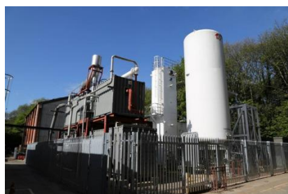
Figure 11. 350 KW/2.5 MWh LAES pilot plant at Birmingham [59].
