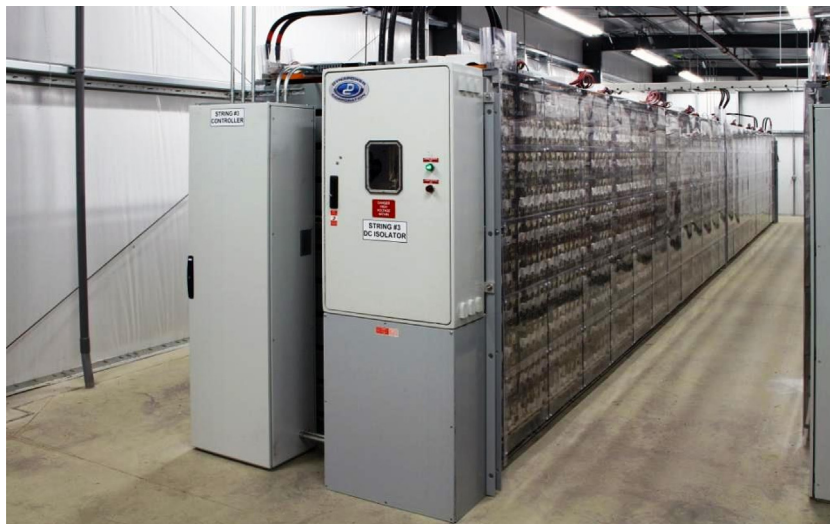
Fig. 10. Lead-based Ultrabattery ® used for frequency regulation at Lyon Station, Pennsylvania.
