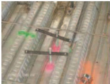
Figure 25: Visual control with color coding to show locations for sheet metal straps and pipe hangers in metal decking (Figure 2 in Tommelein 2008, source: John Mack, Southland Industries, Inc., presentation at 2007 Annual Conference of the Lean Construction Institute, San Francisco, CA)
