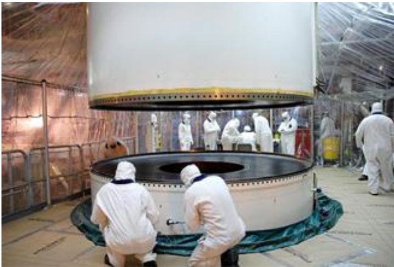
Figure 2. In a Vehicle Assembly Building high bay, an aft center segment of a Solid Rocket Booster is lowered toward a segment already in place. Credit: NASA
