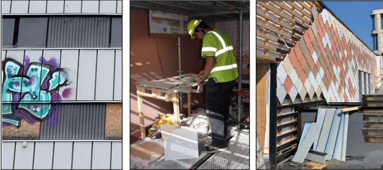
Photo from inspection, Oppsal nursing home. Photo: Randi Lunke Cutting and assembly work. Photo: Anne S Nordby Facade panels during installation. Photo: Randi Lunke
