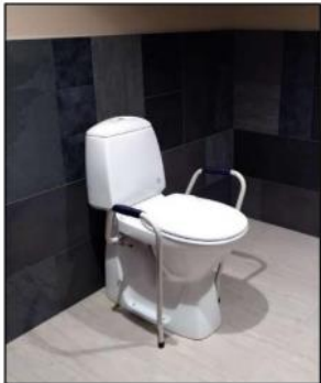
Sanitary equipment in the original building, under storage and installed in KA13. Photo: Anne S Nordby
