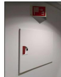
Used fire hose cabinet from DEGS mounted in KA13. Photo: Anne S Nordby
