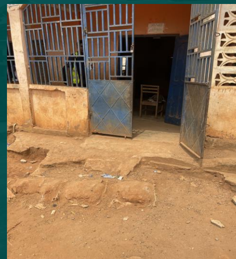
➤ Image showing the depleted state of classroom entrance
