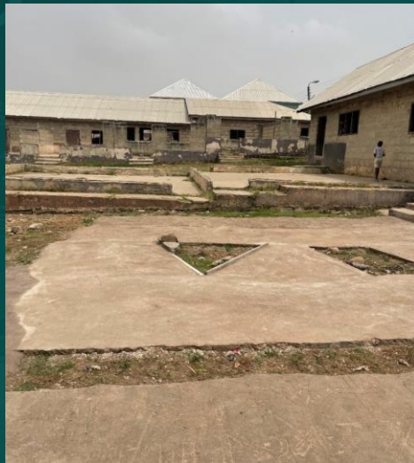
➤ Image showing depleted state of flooring
