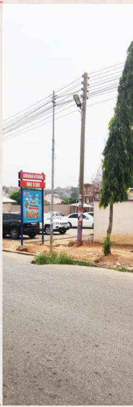
Exposed Cables across streets
