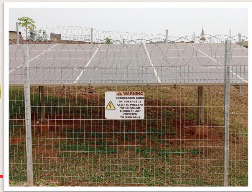
Solar system at shell fuel station near the Kumasi central mosque.
