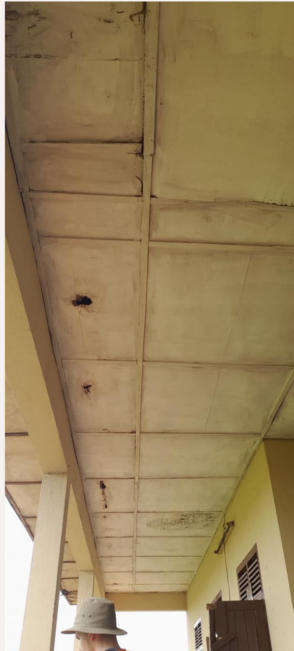
Poorly maintained plywood ceiling
