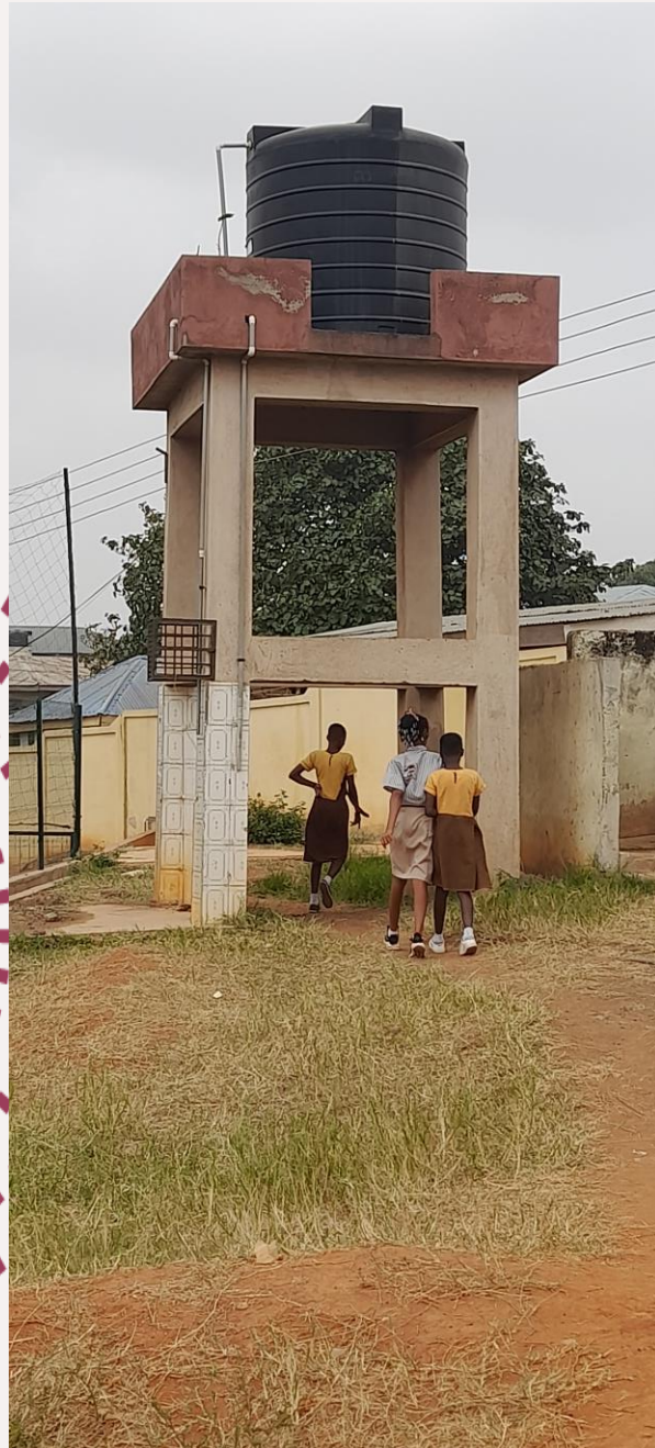
Water Storage Tank
