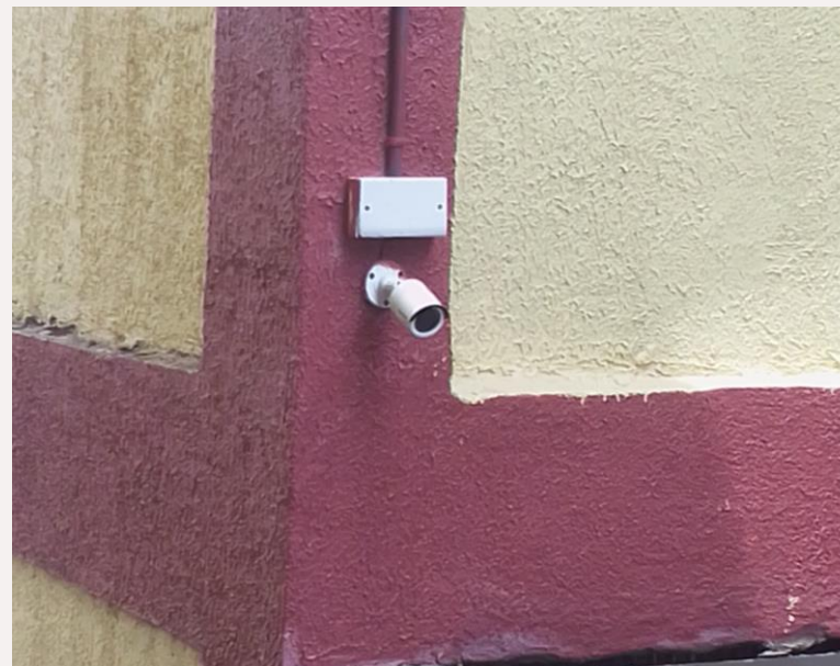
CCTV Security Camera
