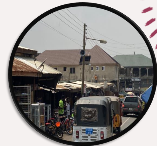
P.A system on street light pole
