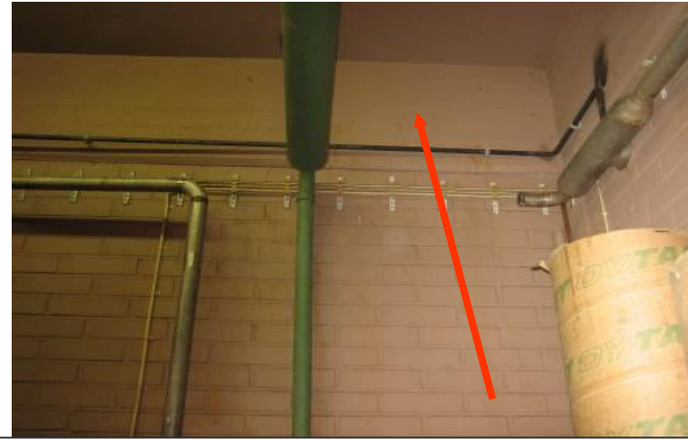
Location of the removed pipeline section between tap water and waste water lines
