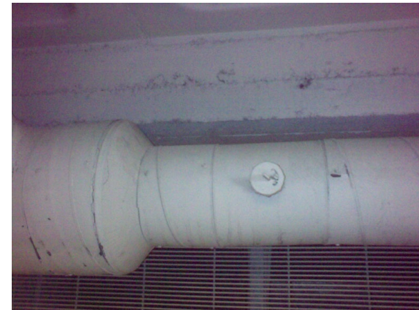
Transition is too steep.
