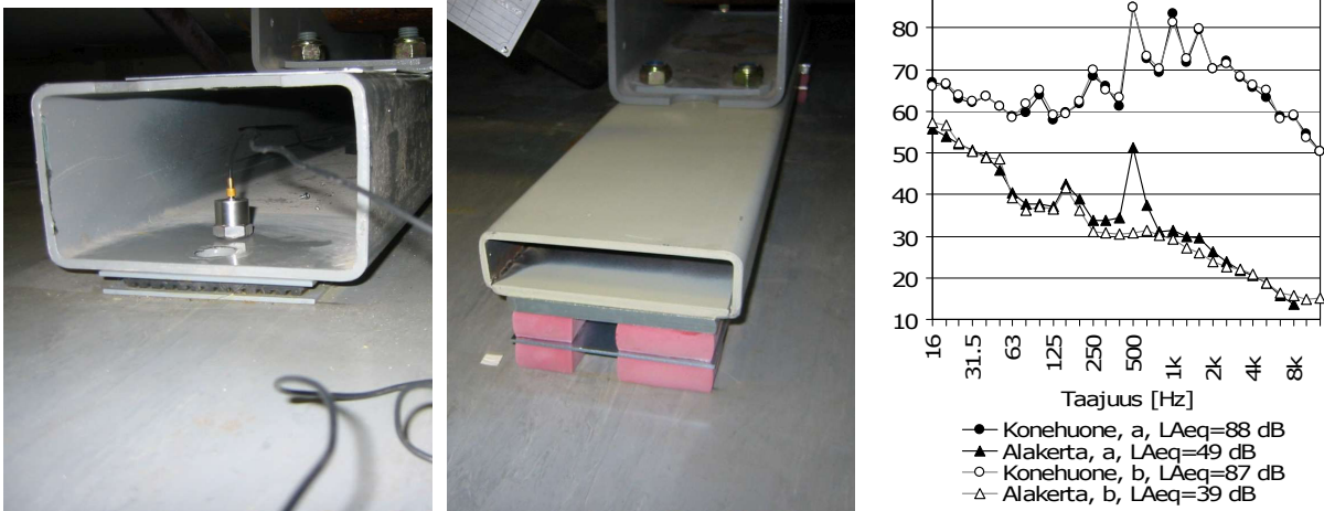
Fig. 11.6.3. The photographs show elastic vibration insulation between the frame and floor of the steel unit. (a) The wrong type of vibration isolator that does not compress sufficiently. (b) The correct type of vibration isolator with sufficient compression. (c) SPLs in the engine room and below office for each type of insulator. The type b insulator achieves the desired attenuation at 500 Hz.
