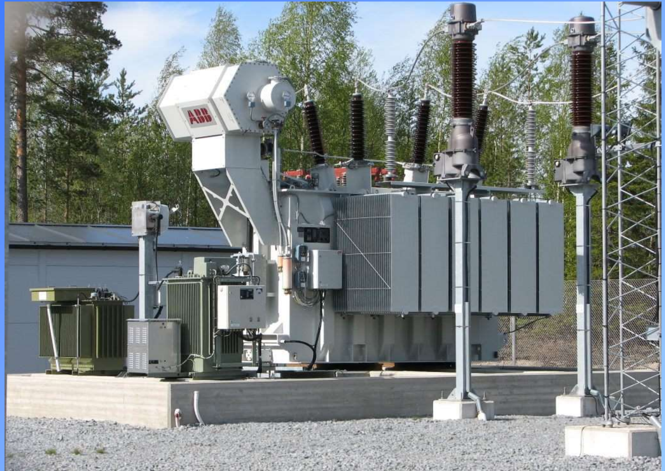
110 kV / 20 kV primary transformer
