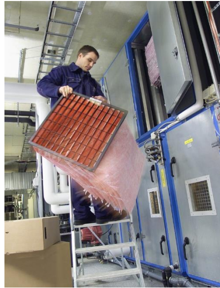
Air filter in air handling unit.
