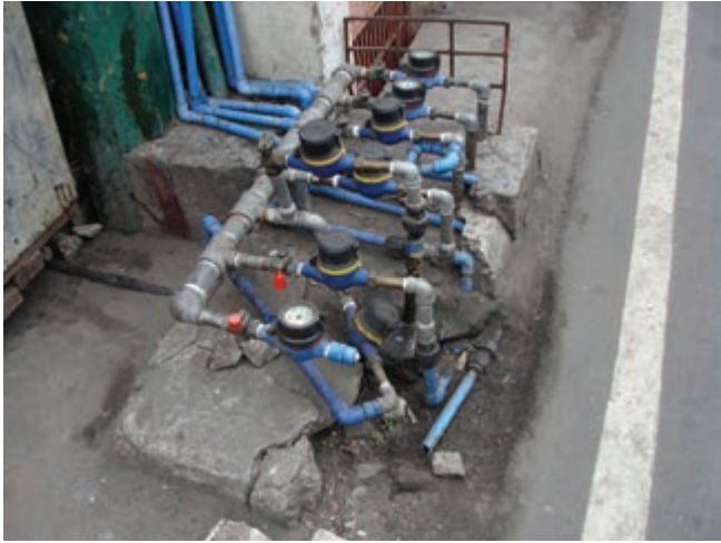
Manila, Philippines Exposed gas valve pipes and meters.
