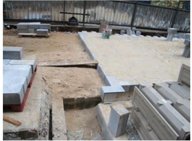
São Paulo, Brazil Drainage channels under construction for a street repaving project.
