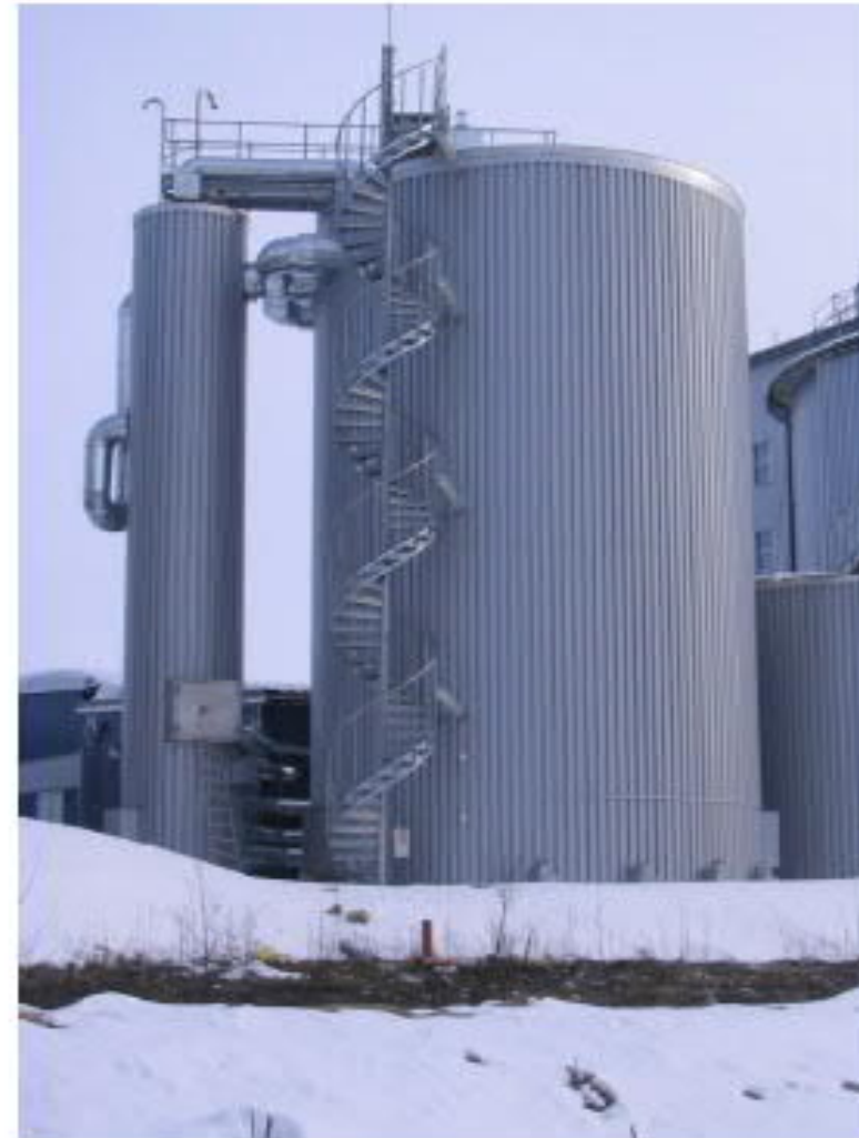
Typical Biobed® EGSB plant at Lapin Kulta, Haparanda (Finland)
