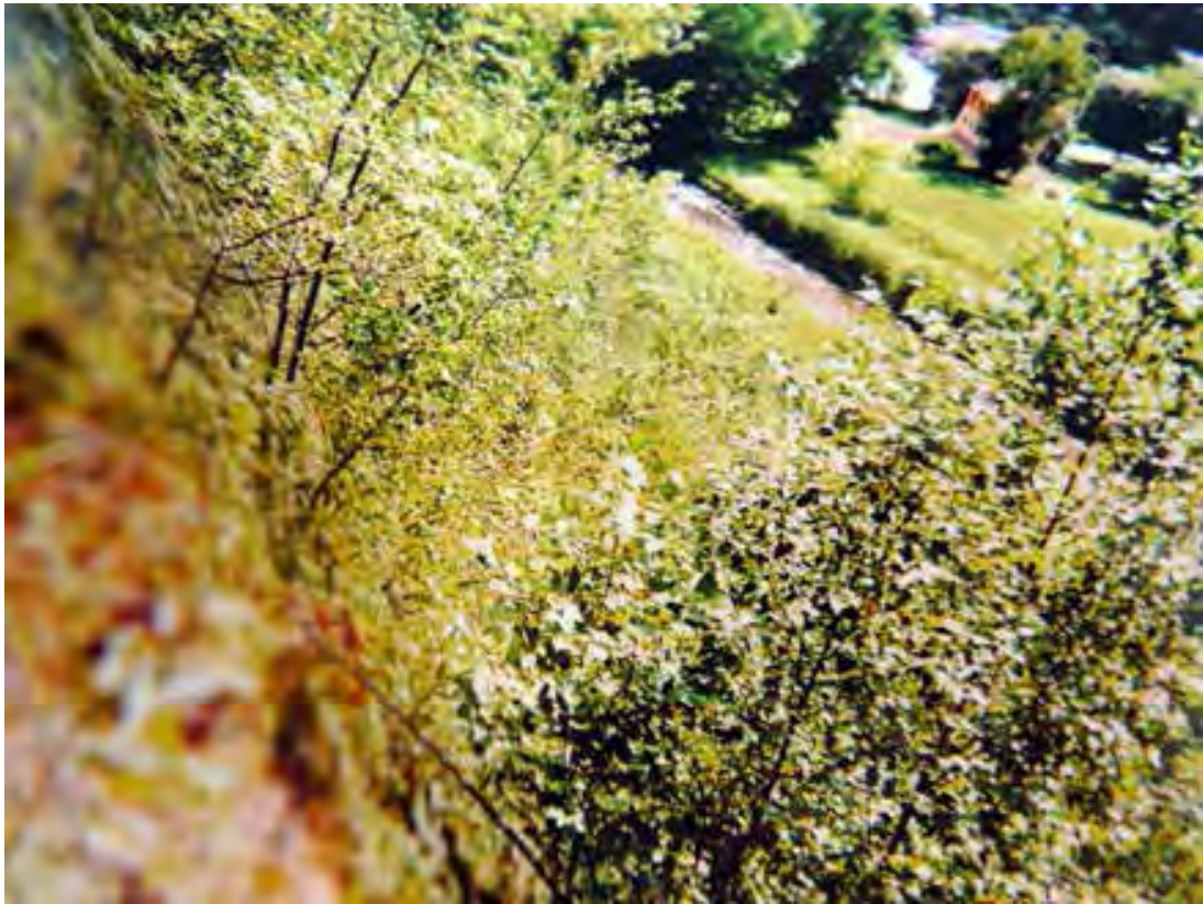
Fig. 04 DISCONTINUITY/UNSTABLE MATERIAL Deer Run Heights, site of 1999 Jeffersonville landslide 44°38'45.54"N 72°49'27.53"W
